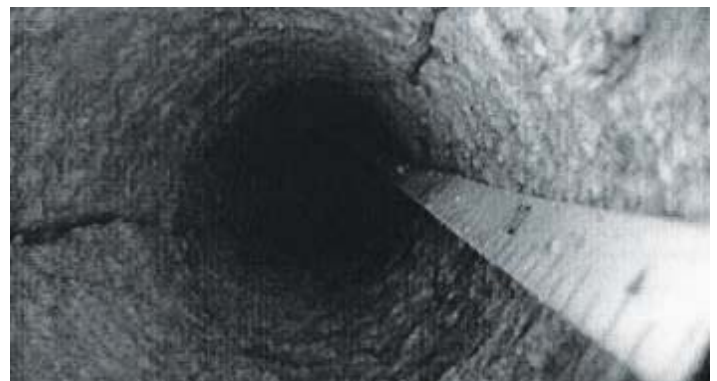
Figure-7 Image inside monitoring drillhole showing cracks (Brent and Smith 6 )
