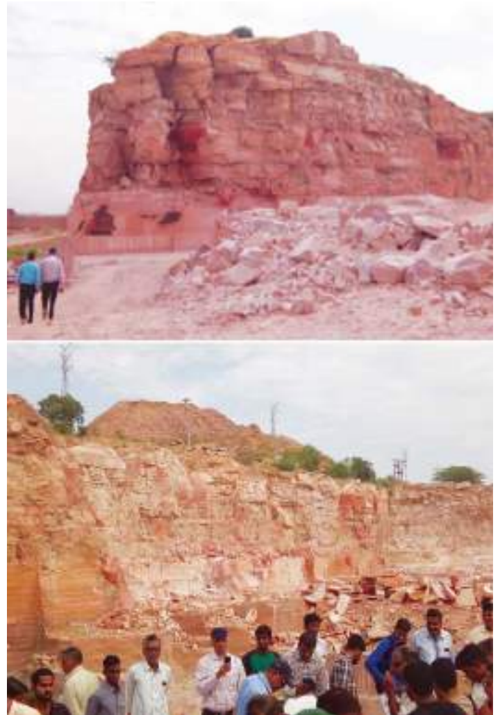
Fig.11 A Sandstone mine with near vertical cliff: Prone to roll down
