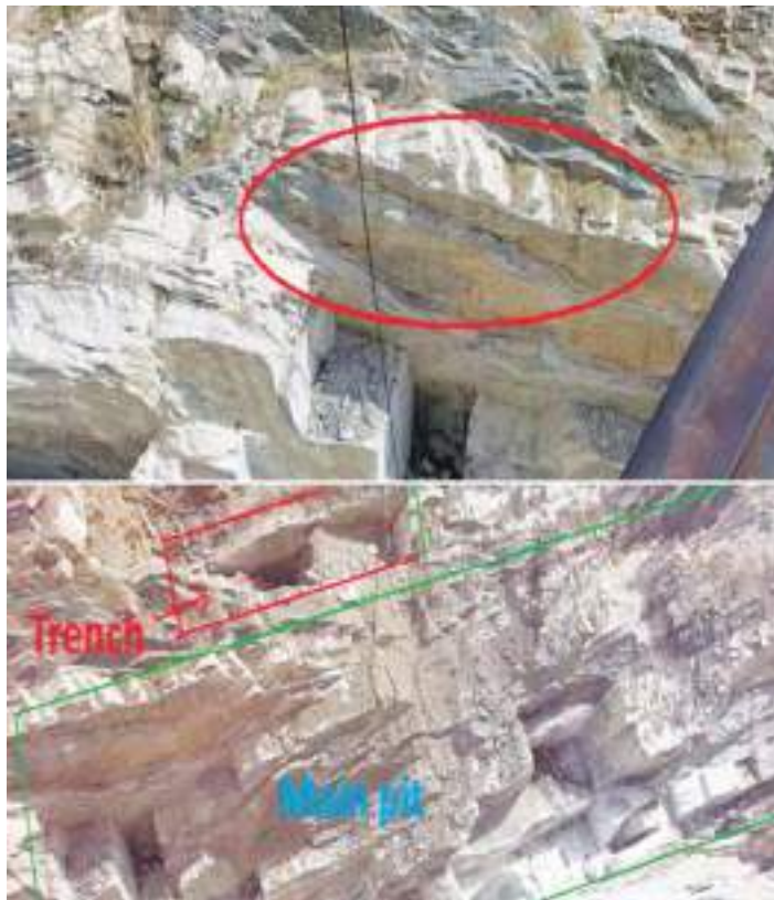
Fig.9 Development of cracks and creation of trenches in the hangwall of the mega-pit of Makrana
