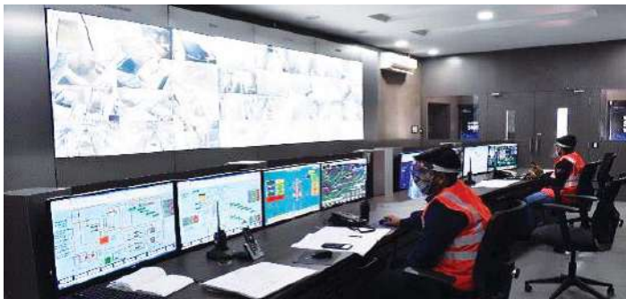
Fig 21: Integrated operation center (IOC) & Integrated Remote Supervision Center
