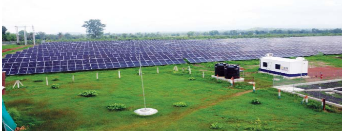
Solar power plant: a step towards Renewable Energy
