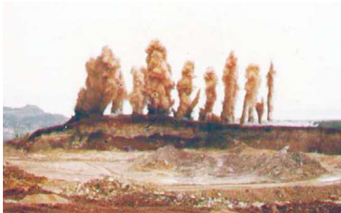
Figure 8 - STEMMING EJECTION (RIFLING) (Photo by IDL Industries Ltd - Technical Services)
